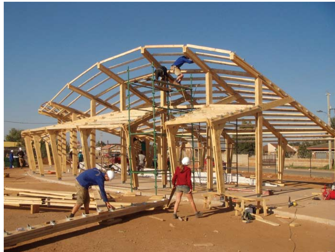
Frames prefabricated by students in a local building yard were erected by crane and the frame was completed a bay at a time. Test runs for prefabrication were carried out in Nottingham to prove the construction method. Photo: John Edmonds
